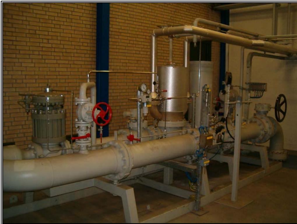
Figure 1: example of an industrial gas installation
